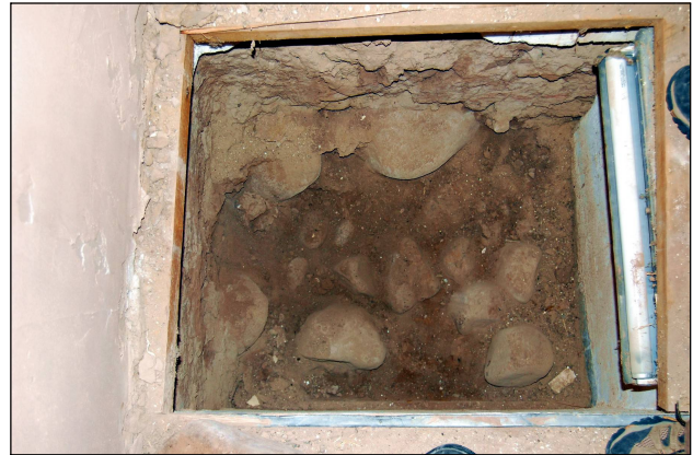
Portion of the original foundation and wall from the 1620s pueblo built mission church.
