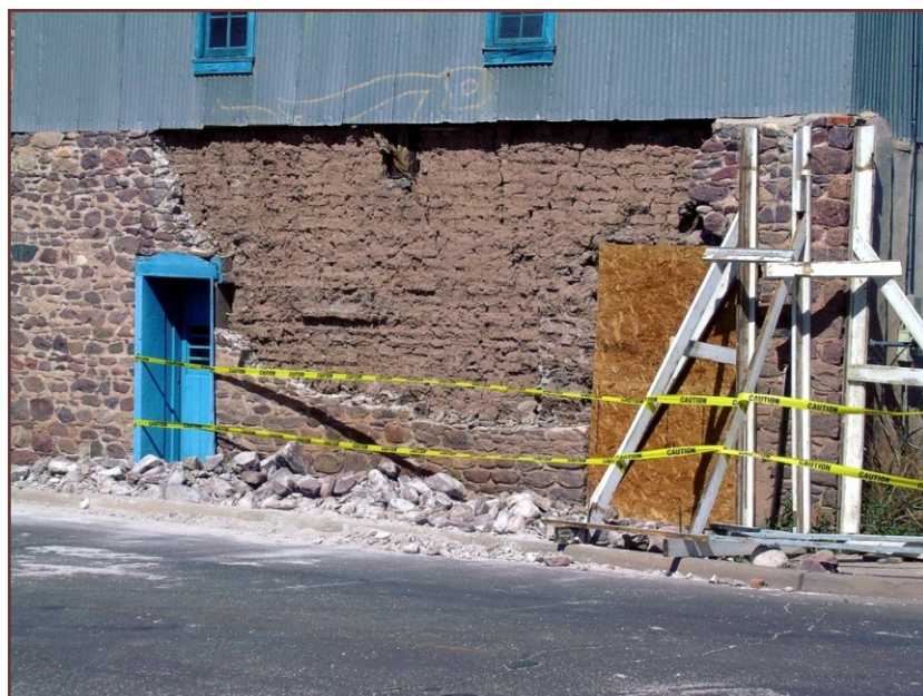
The collapsed wall on the Hammel Museum
