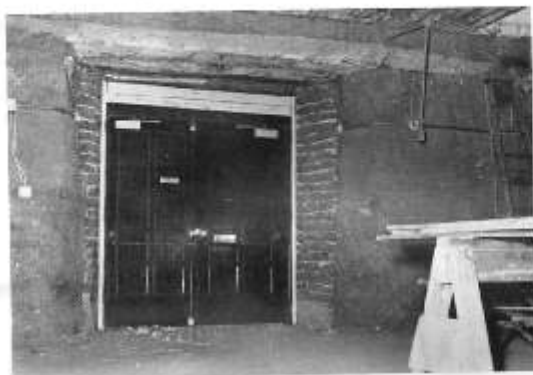
Main Entrance with plaster removed. Note different types of adobes, uncovered lintels, and Choir floor.
