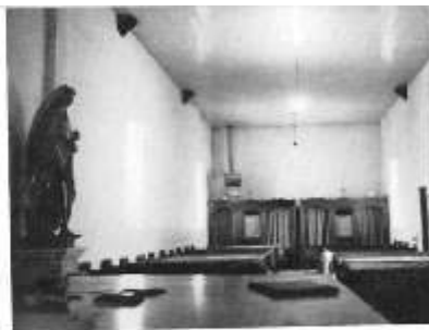
The stained ceiling the extent of lighting!
