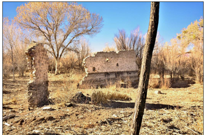
View looking west at Foreman's shack wall (left) and roundhouse wall (center).
