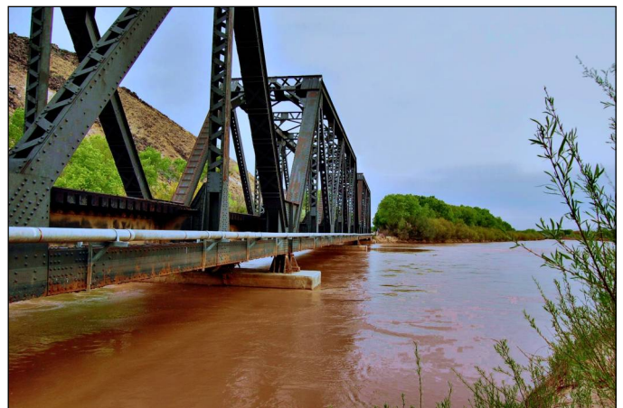
Mainline trestle across the Rio Grande, looking south, the entrance to the Jornada del Muerto and higher ground. Bridge was raised 8 feet after 1929 flood. AT&SF milepost 1005.8
